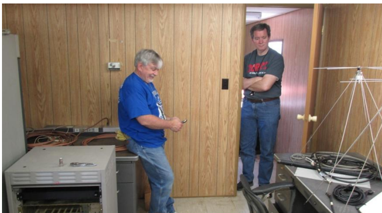
Jon Brown – WB5KSD and Scott Davis – KK7JS getting coax cables in order to tie the new transmitter to existing duplexers.
