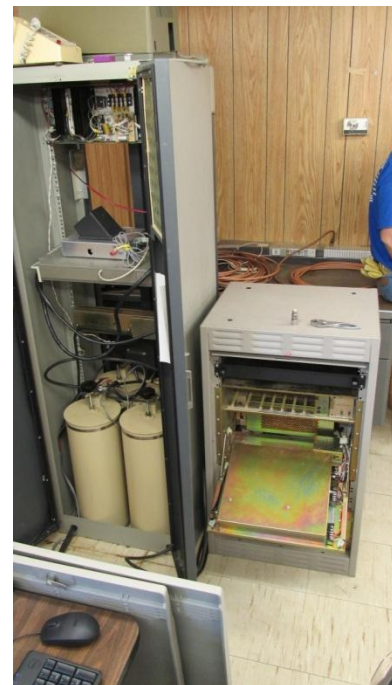
The new GE Mastr II is in the small cabinet on the Right of the existing cabinet.
