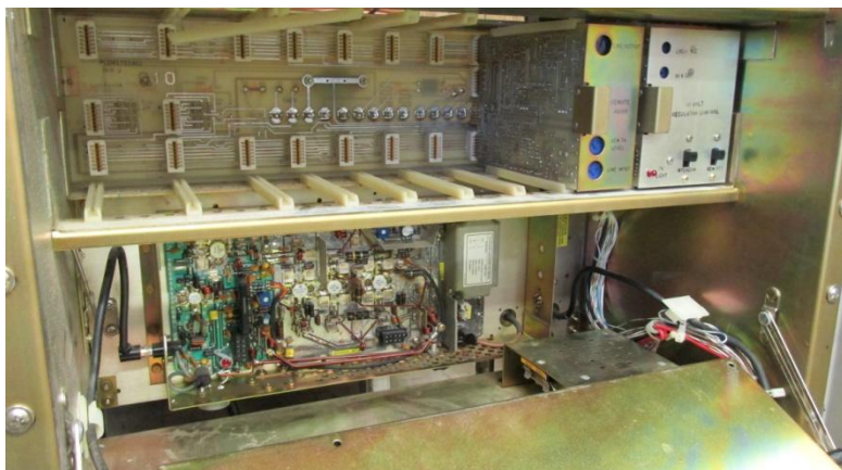
Inside the transmitter of the new GE Mastr II Base Station.
